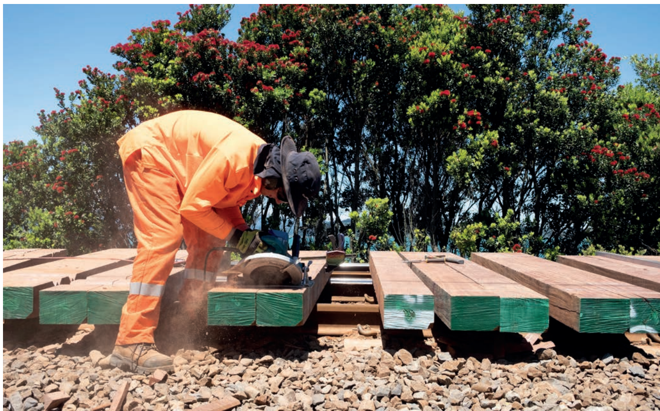
Tailoring replacement sleepers for a bridge on the North Island Main Trunk near Wellington.
