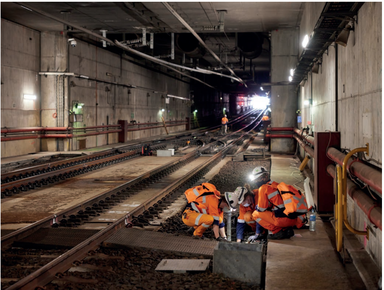
KiwiRail is progressively preparing Britomart for the opening of the City Rail Link.
