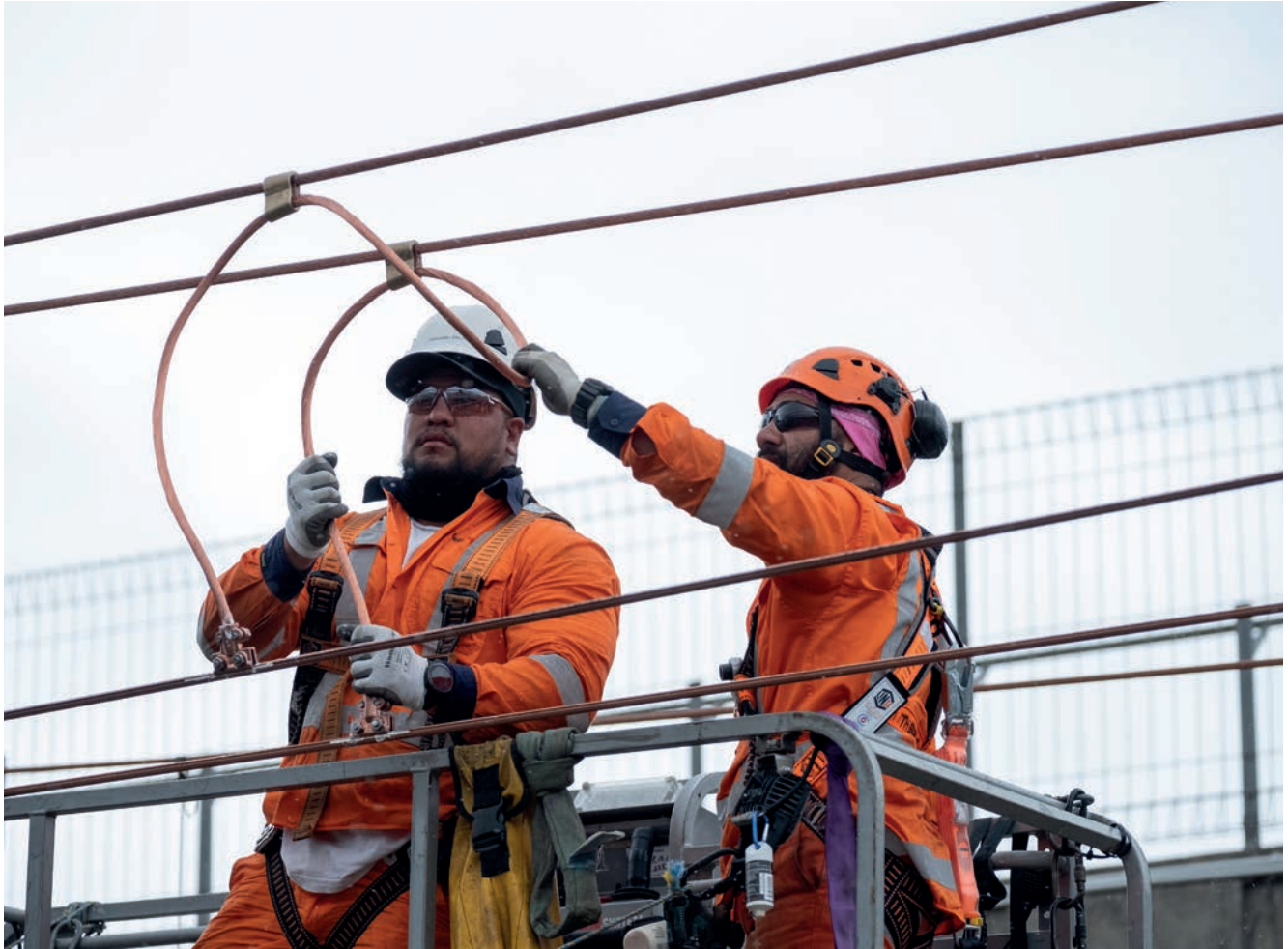
Renewing the overhead power supply on commuter lines is part of network maintenance.
