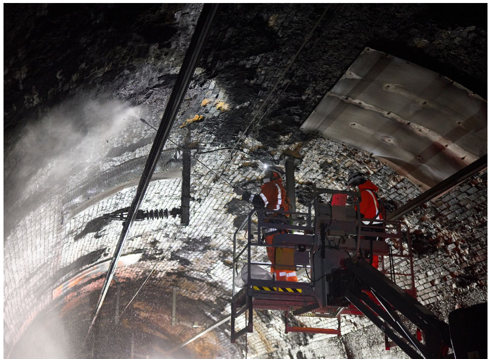
Recent water blasting of the Parnell Tunnel reveals where repairs need to be made
