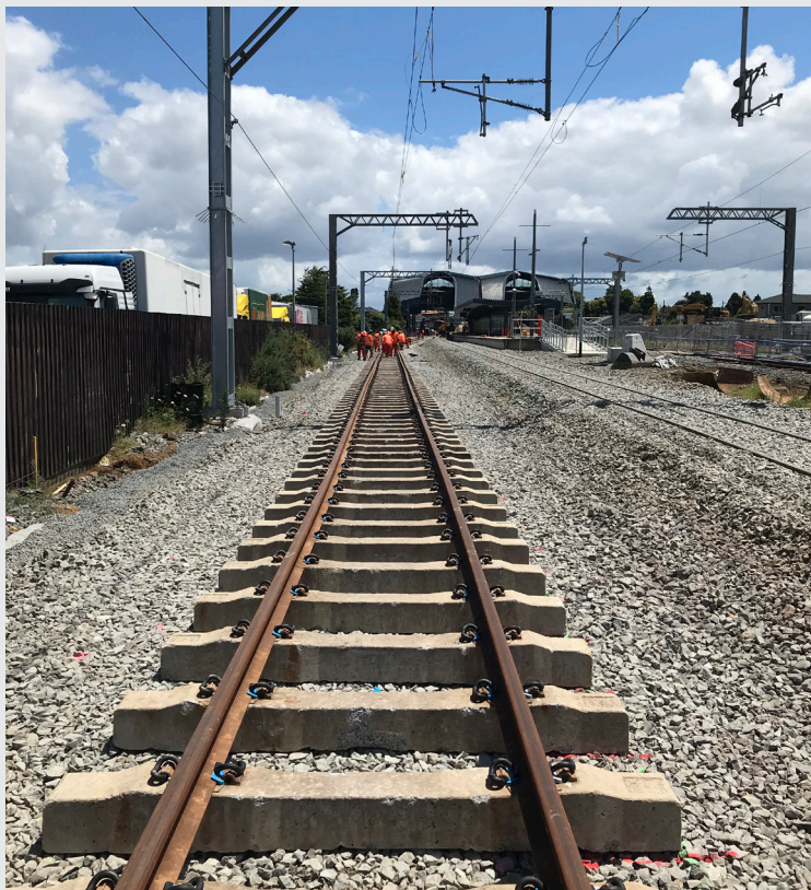
This section of track south of Puhinui Station was moved sideways a few metres as part of the Third Main Track project.
