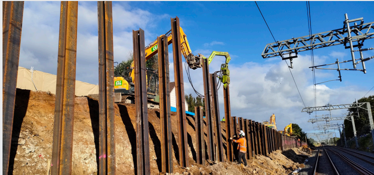
Building a retaining wall just north of Puhinui Station for the Third Main Track project
