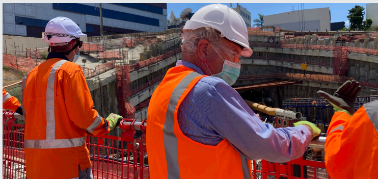
New Chair David McLean (right) at the entrance to the City Rail Link tunnel at Mt Eden Station
