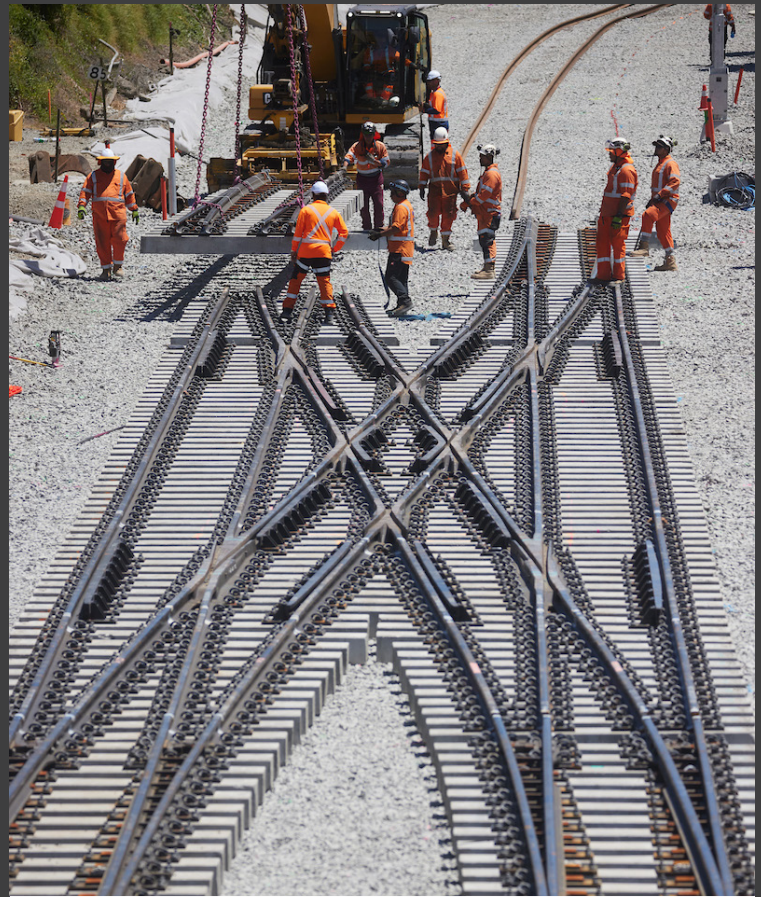
The new scissor crossover at Pukekohe Station. This track structure, allows trains to move from one track to another
