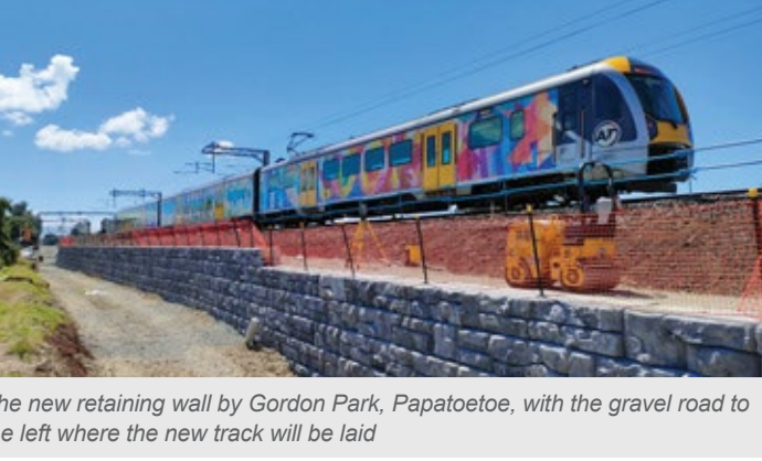
The new retaining wall by Gordon Park, Papatoetoe, with the gravel road to the left where the new track will be laid
