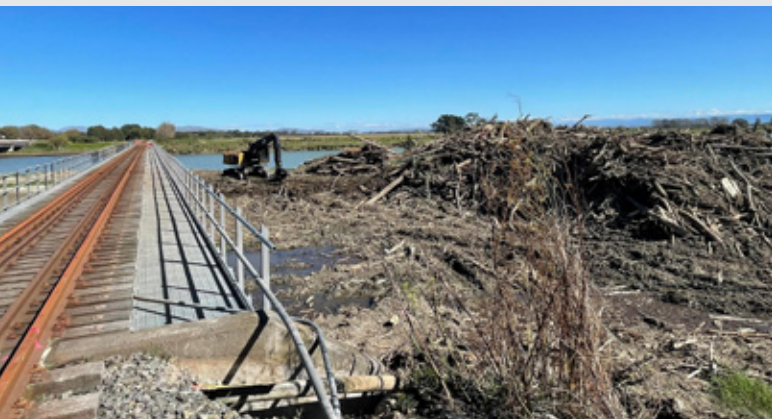
Wood debris being cleared from a rail bridge in Awatoto
