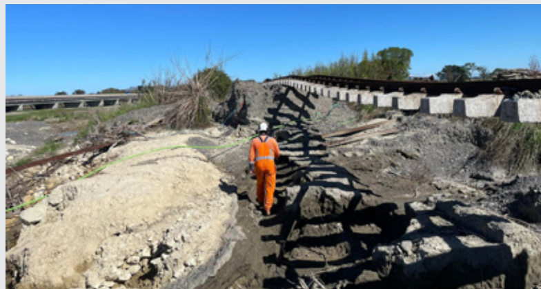
Flood damaged tracks around Awatoto
