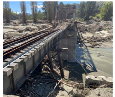
Damage to a bridge in Esk Valley
