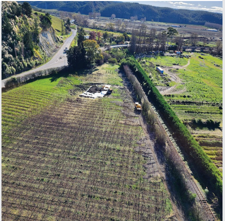
'Make safe' work between Napier and Wairoa - clearing ballast that had washed off the rail line, blocking culverts, in Bayview
