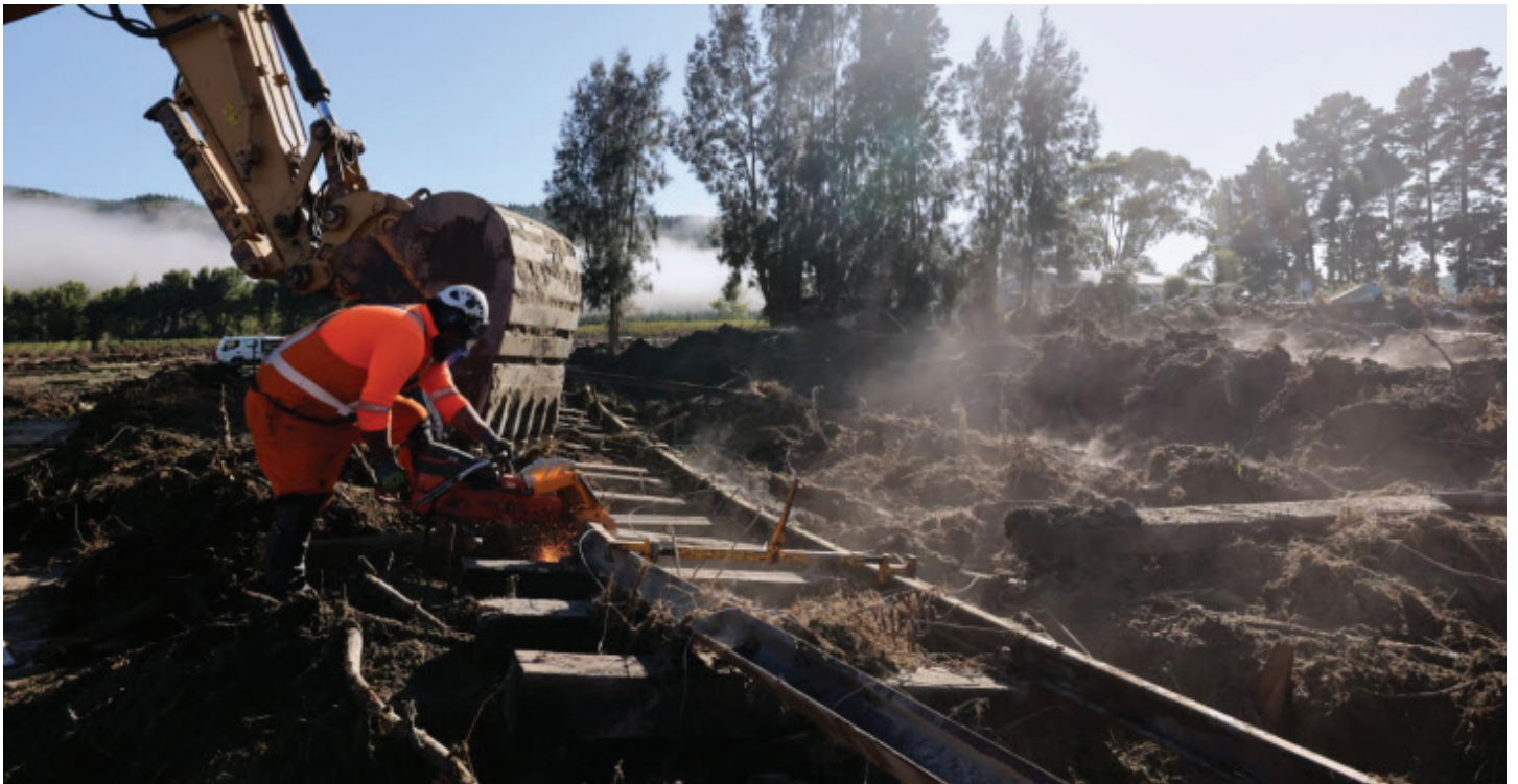
Removing damaged rail in Eskdale. The digger is holding the rail down while the person cuts it
