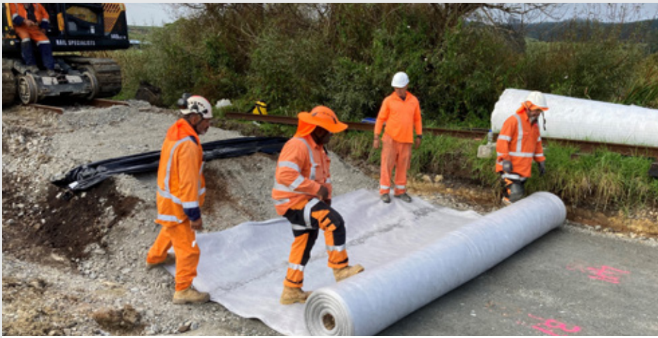
North Auckland - laying down geotech cloth prior to laying ballast at Woodhill
