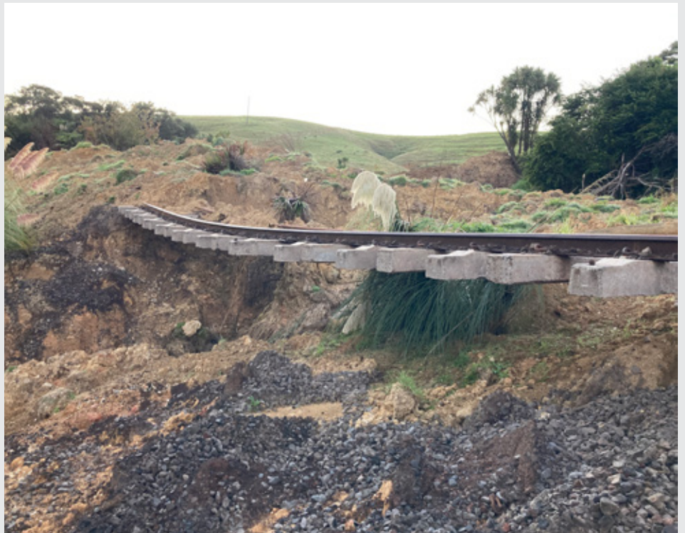
North Auckland - slip covered rail line at Tahekeroa
