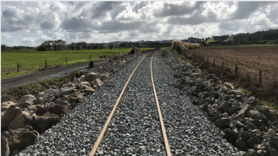
North Auckland - repaired line with rock protection after washouts south of Helensville
