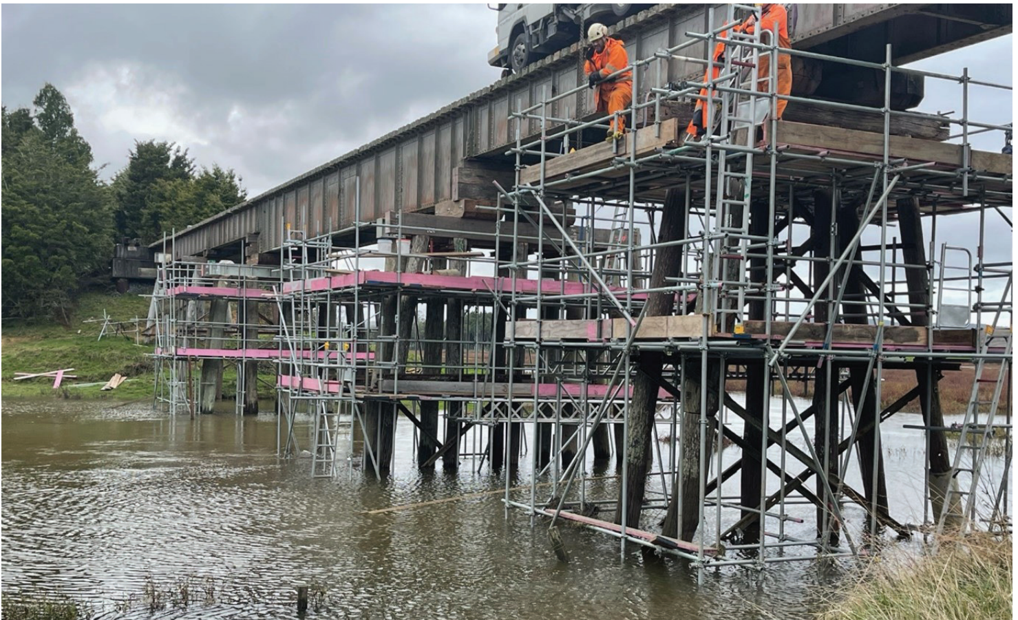
A range of work is being undertaken on Bridge 150 at Paparoa, including on piles and corbels.
