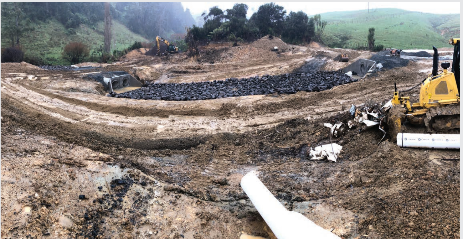
Completion of the graded rock apron in the basin between the road (right) and rail (left) culverts. A large amount of landslip material had to be removed from this area.
