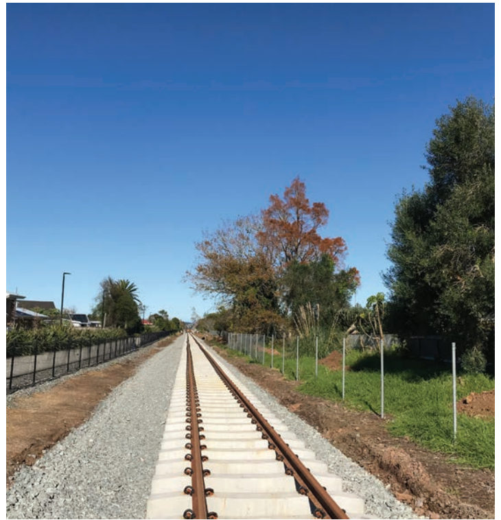
Track laid on ballast bed between Kensington and Kamo Road crossings in Whangārei
