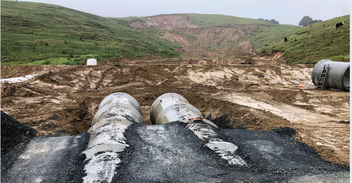
Road culverts being installed. The road bund and new road, will be built on top of them. See the temporary earth bund, to protect the site during construction, and the scarred hillside in the background.
