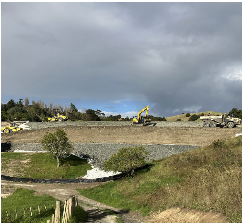
147km rebuild nearing completion, where a huge slip below the rail line caused a 100-metre embankment to fail. About 21,000 cubic metres of saturated material had to be excavated and the embankment rebuilt.
