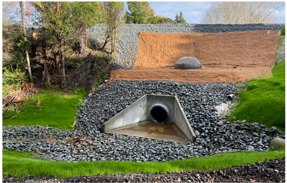
An example of erosion control - improved drainage around the 99km mark, near Woodcocks.
