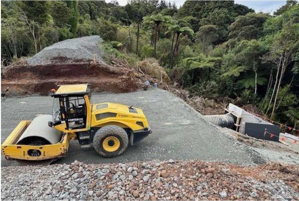
Work progressing at the massive 223km washout site south of Kauri, with a large culvert now installed.
