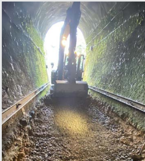
During this year’s weather events slips fell down across both ends of Tunnel 1. At the northern end large amounts of water carried sediment into the tunnel, ruining the ballast that the tracks sit on. Forty metres of track inside the tunnel was removed and the affected ballast excavated, down to the track foundation
