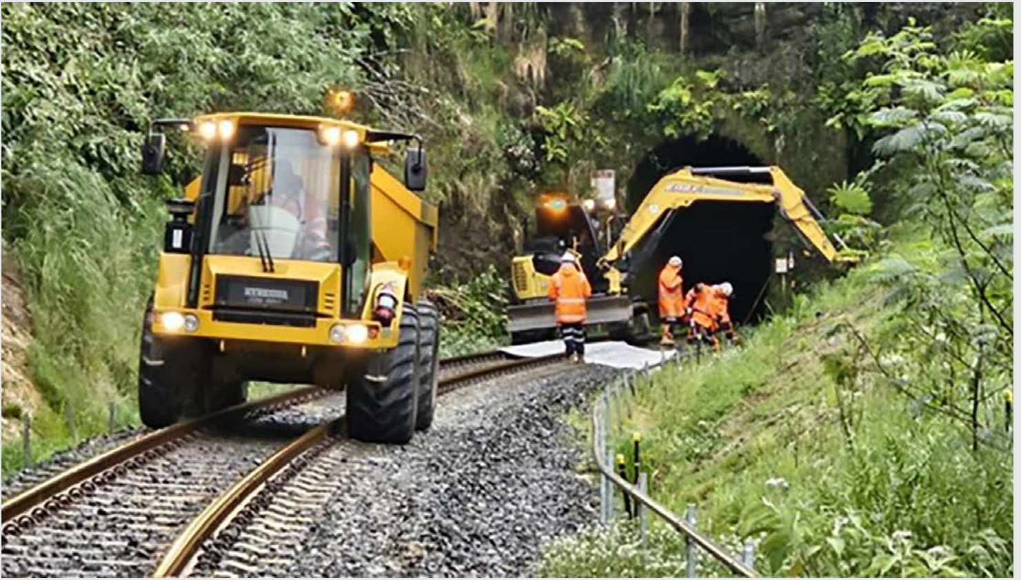
Clearing slips next to the southern entrance of Tunnel 1. The digger is reducing the slope of the bank, which will then be hydroseeded (sprayed with grass seed) to help stabilise it.
