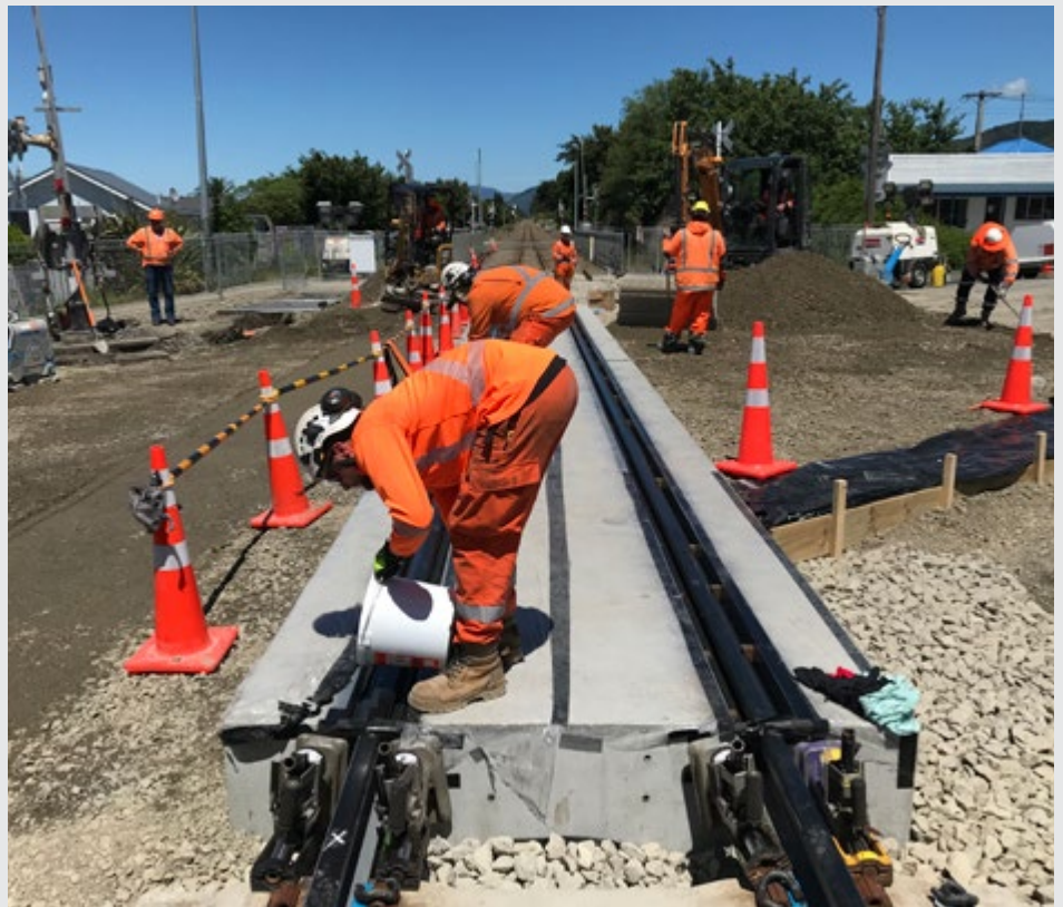
Making safety and performance upgrades to the Fitzherbert St, Featherston, level crossing over State Highway 2 during the Christmas holidays
