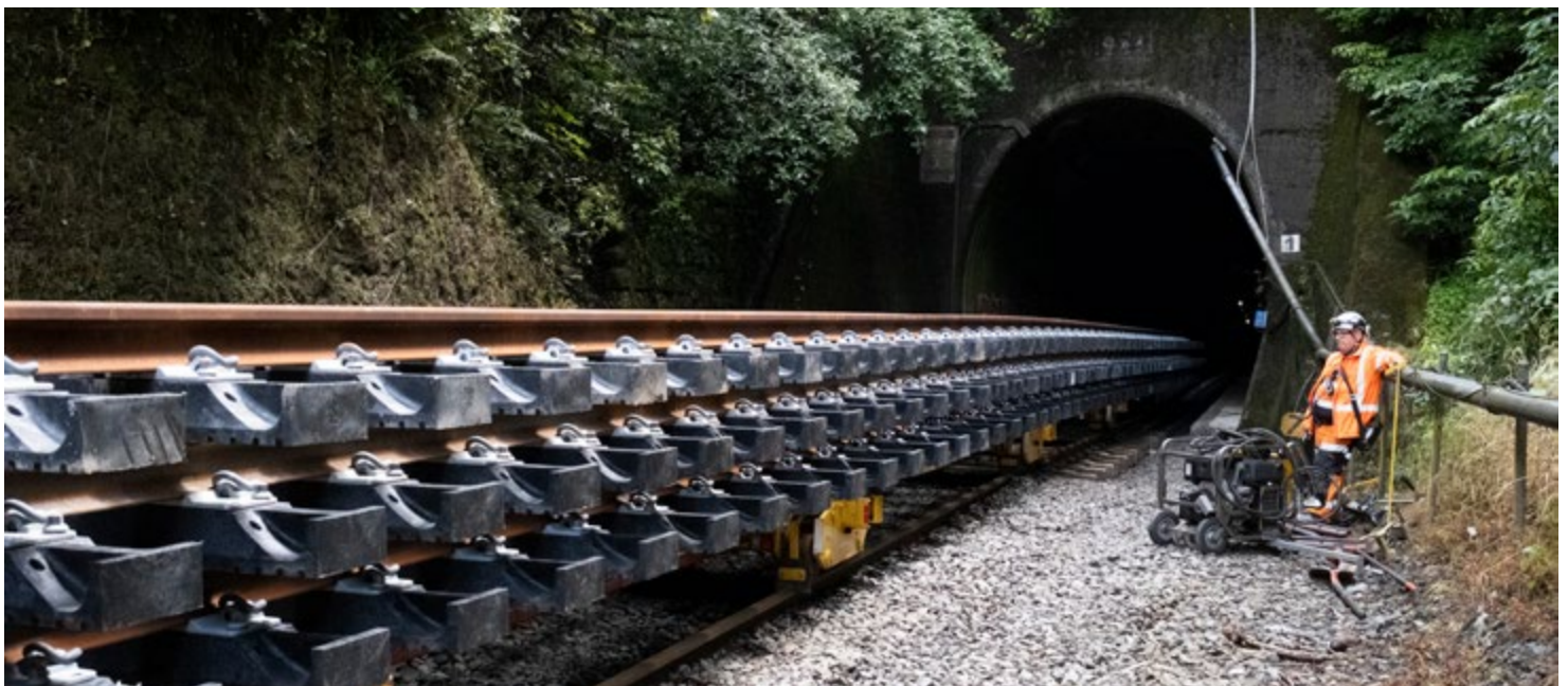
A work train carries 50 metre-long track panels (made up of composite sleepers attached to 50kg rail), for the track replacement in the Maoribank Tunnel over Christmas
