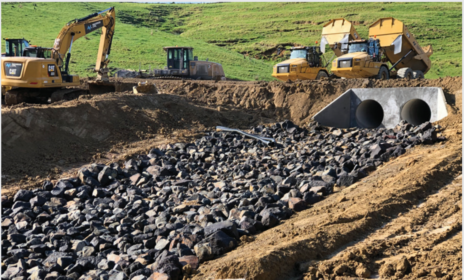
Completion of road and rail culverts and the graded rock apron in the basin between them.
