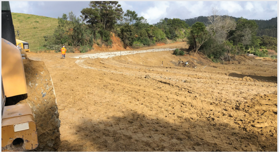
Road embankment under construction – currently approx. 1m cover over the culverts. Lime/cement stabilization has enabled the earthworks to continue through a very wet July.
