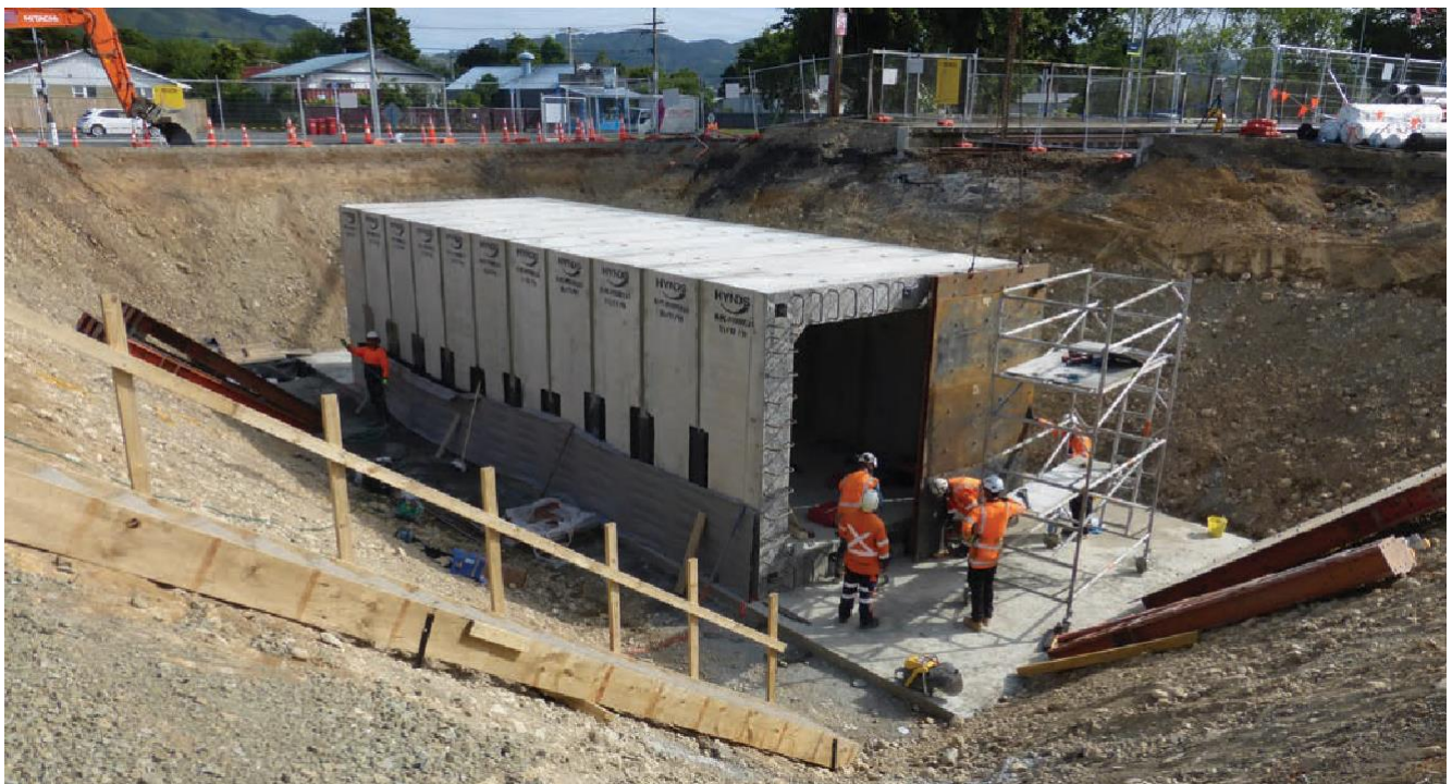
A pedestrian underpass at Trentham is one of the works already completed in Wellington to improve the commuter experience.
