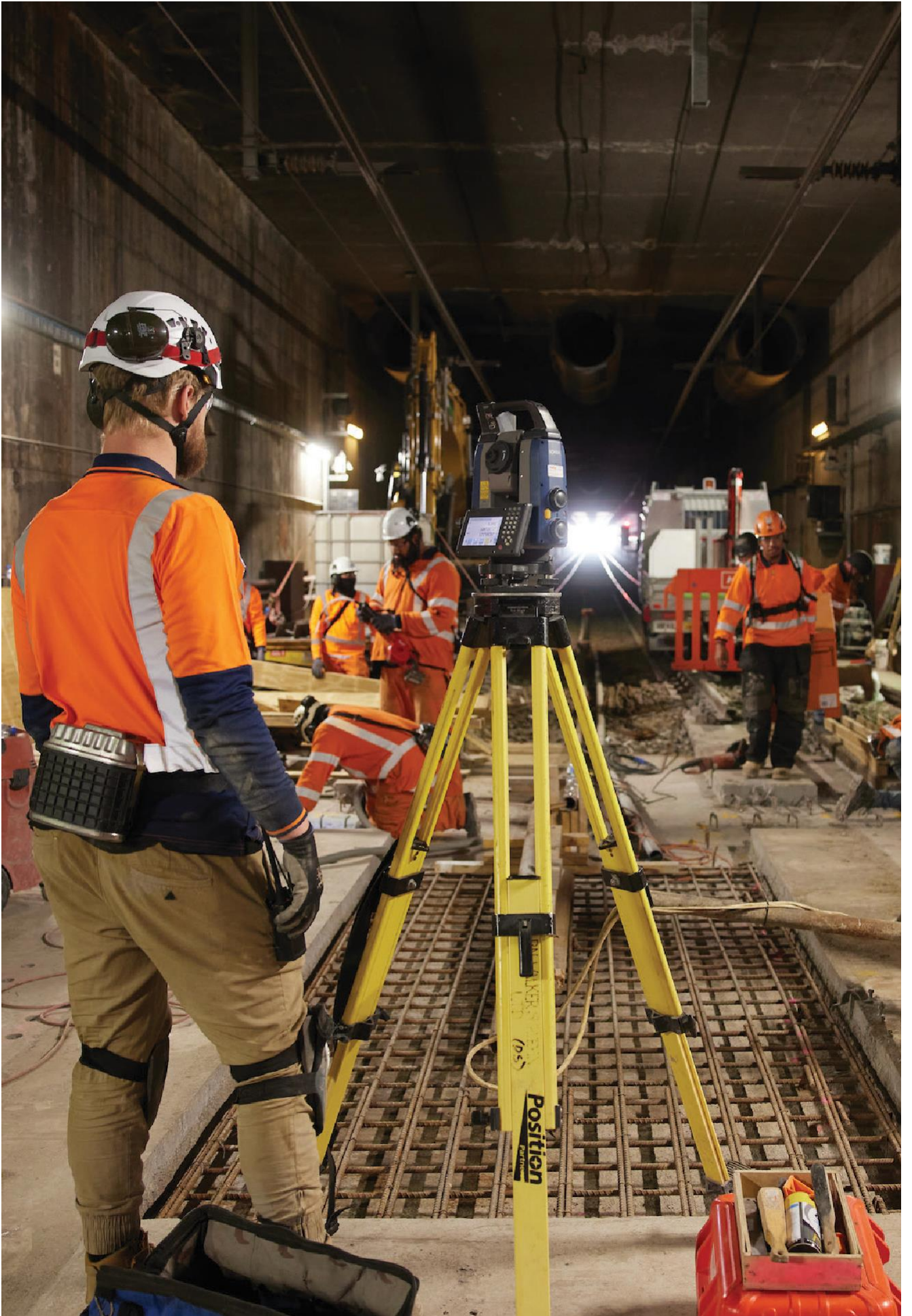
Work underway at Britomart in Auckland. There are specific funding arrangements for metropolitan areas.
