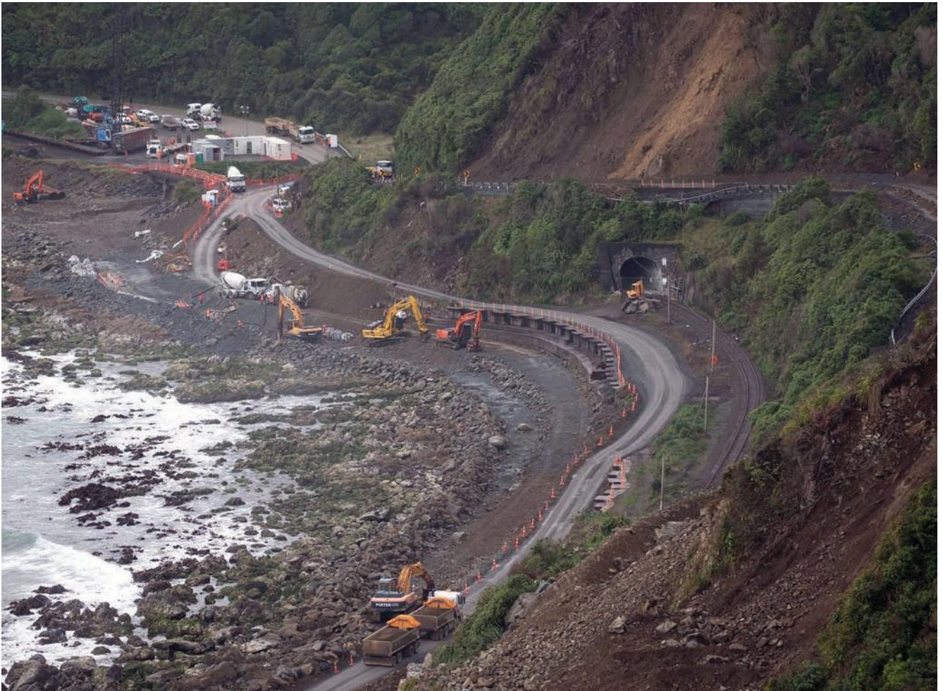
The Kaikoura Earthquake involved major civil works.
