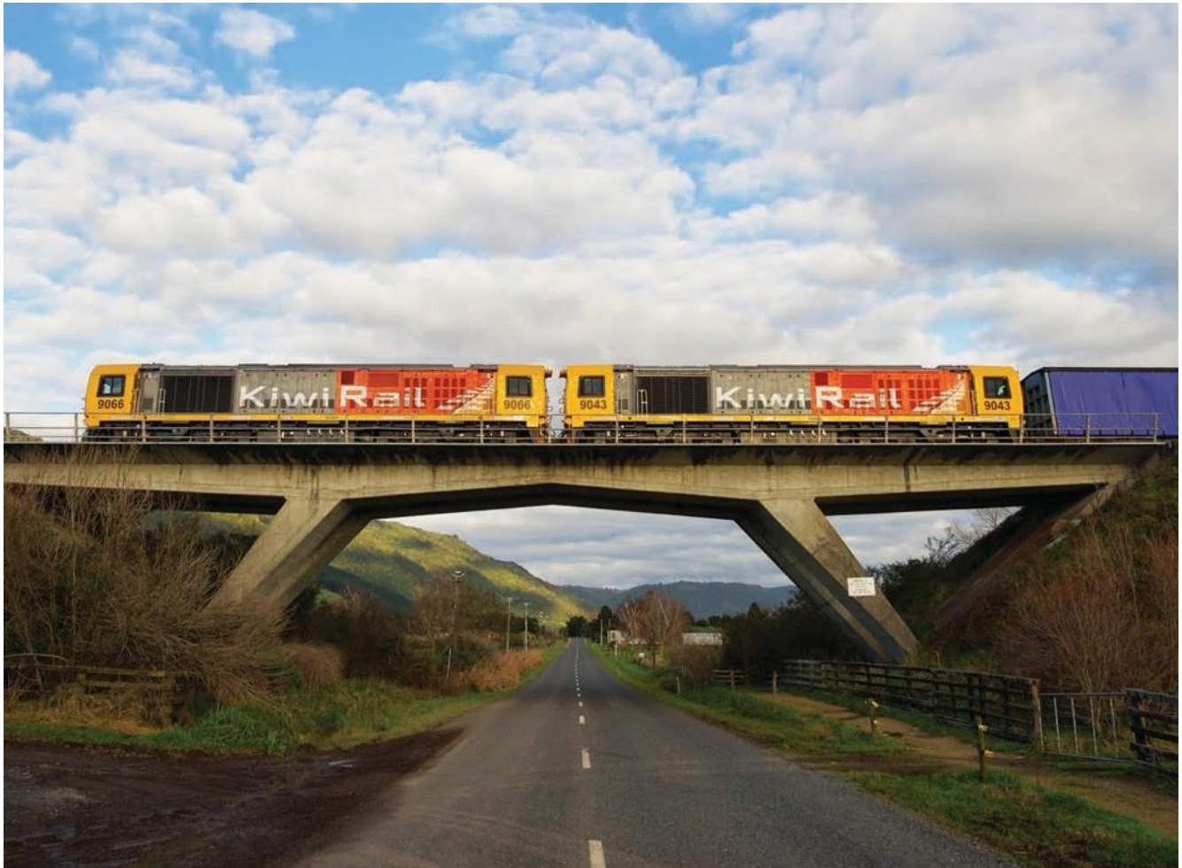
Bridges are key structures for KiwiRail – Bridge 41 on ECMT Kaimai Tunnel deviation.
