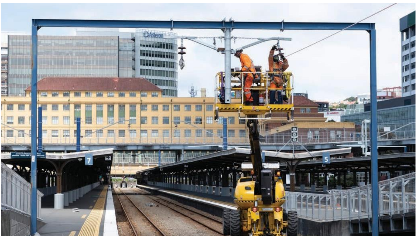
KiwiRail has been working to install modern tensioning systems in the Wellington metro area.
