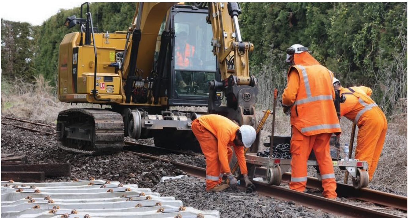
Timber sleepers being replaced with new higher strength and longer lasting concrete sleepers.
