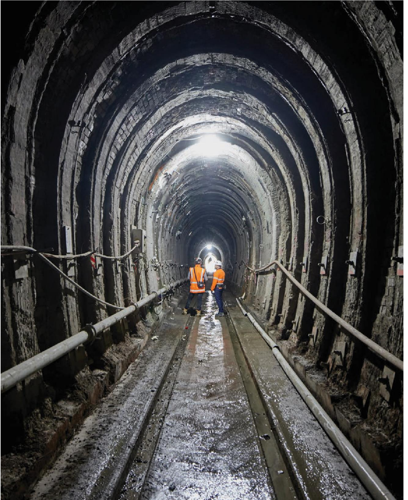
Lowering the floors in tunnels on the Northland line has allowed hi-cube containers to be transported.
