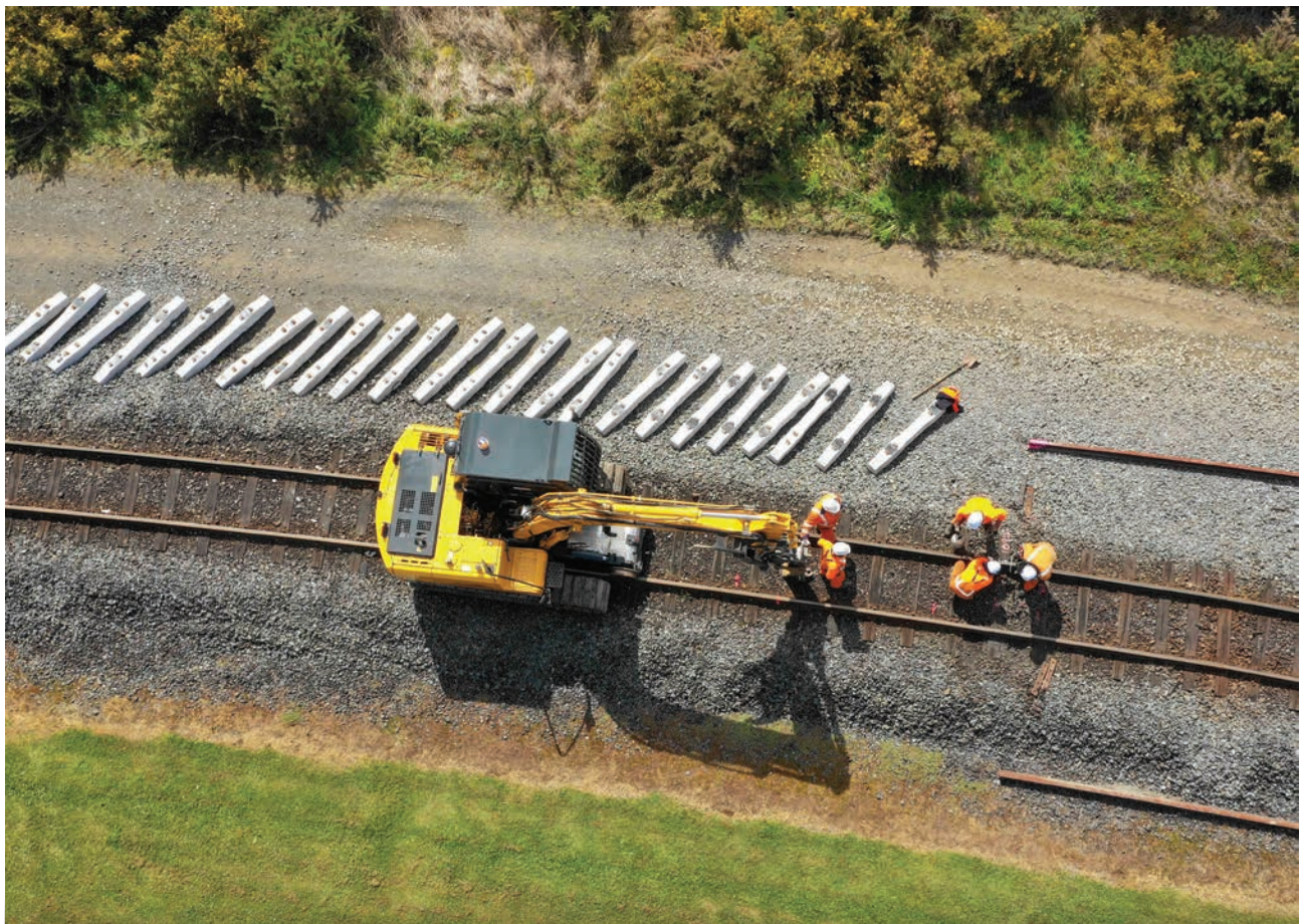
Under the new funding model the national rail network will be funded on a long-term basis alongside the rest of the land transport system.
